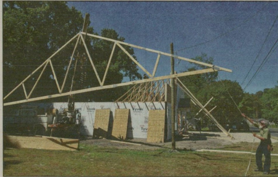
Special to the Crisfield-Somerset County Times/Brice Stump As Harold "Stoney" Whitelock monitors the movement of a truss lifted by his boom truck, Amish builder Mannie Flaud guides the unit into position, with a rope, over the new Skipjack Museum and Cultural Center in Chance as the roof takes shape.
